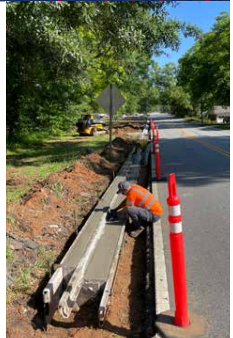
Crew member Eyder Ruiz helps Street Supervisor Chris Smith finish the curbs for additional sidewalk on Hedge Street in June. guys step up and meet challenges head on,” West said.
